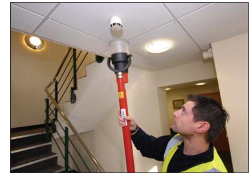
Fig 13 - Service and maintenance in practice
